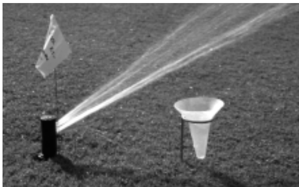
Place the catch can far enough away from the sprinkler head to avoid obstructing the spray pattern.
